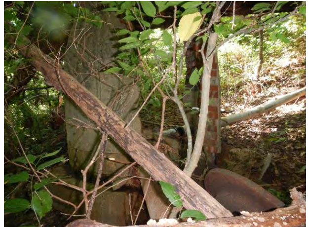
Manhole 12210 collapsed with exposed mains
