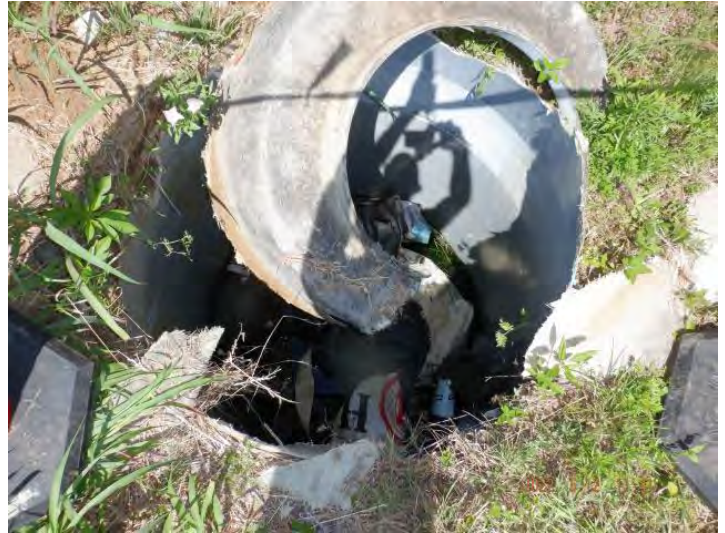
Manhole 24072 – Fiberglass manhole destroyed and full of debris
