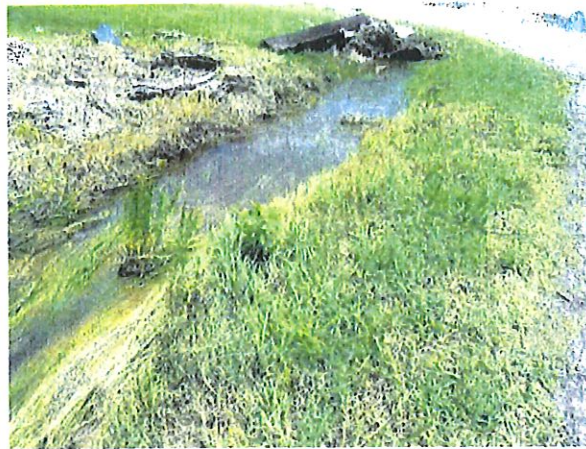
Above: Inadequate drainage in a swale from 2017
