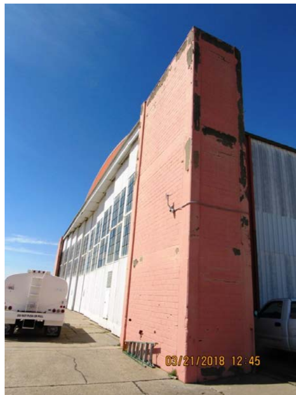
Fuel Truck Adjacent To Southeast Hangar Door System
