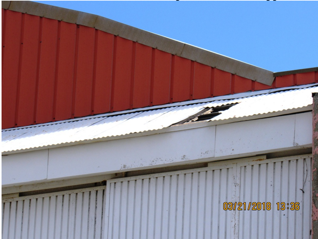
Minor Damage To External Paneling Above Hangar Door
