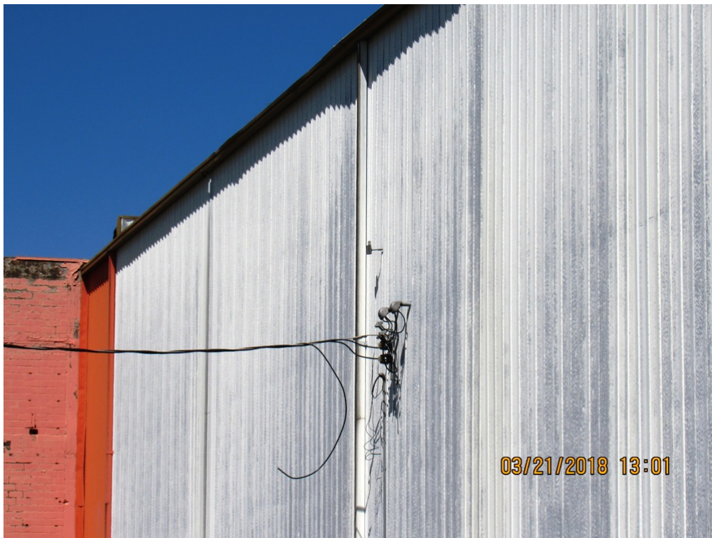
View Of External Wall System Showing Electrical Connection
