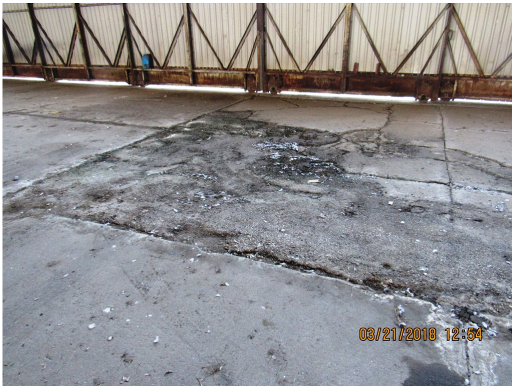
View of Interior Floor System Showing Deterioration and Spalling
