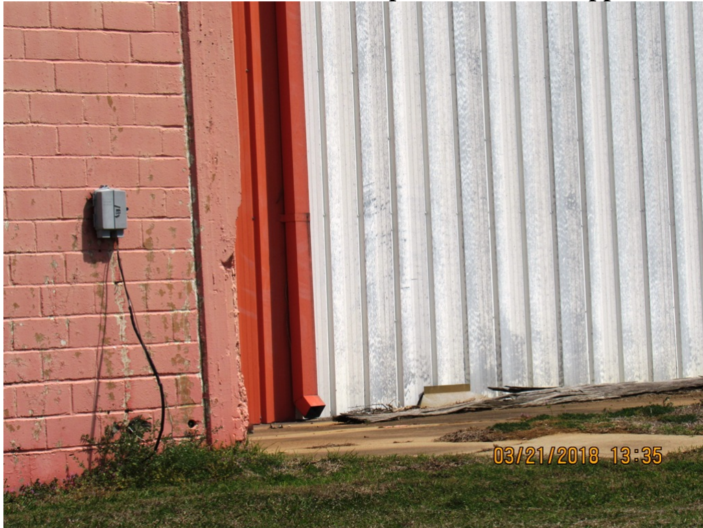
Gutter And Downspout System Adjacent To Hangar External Wall
