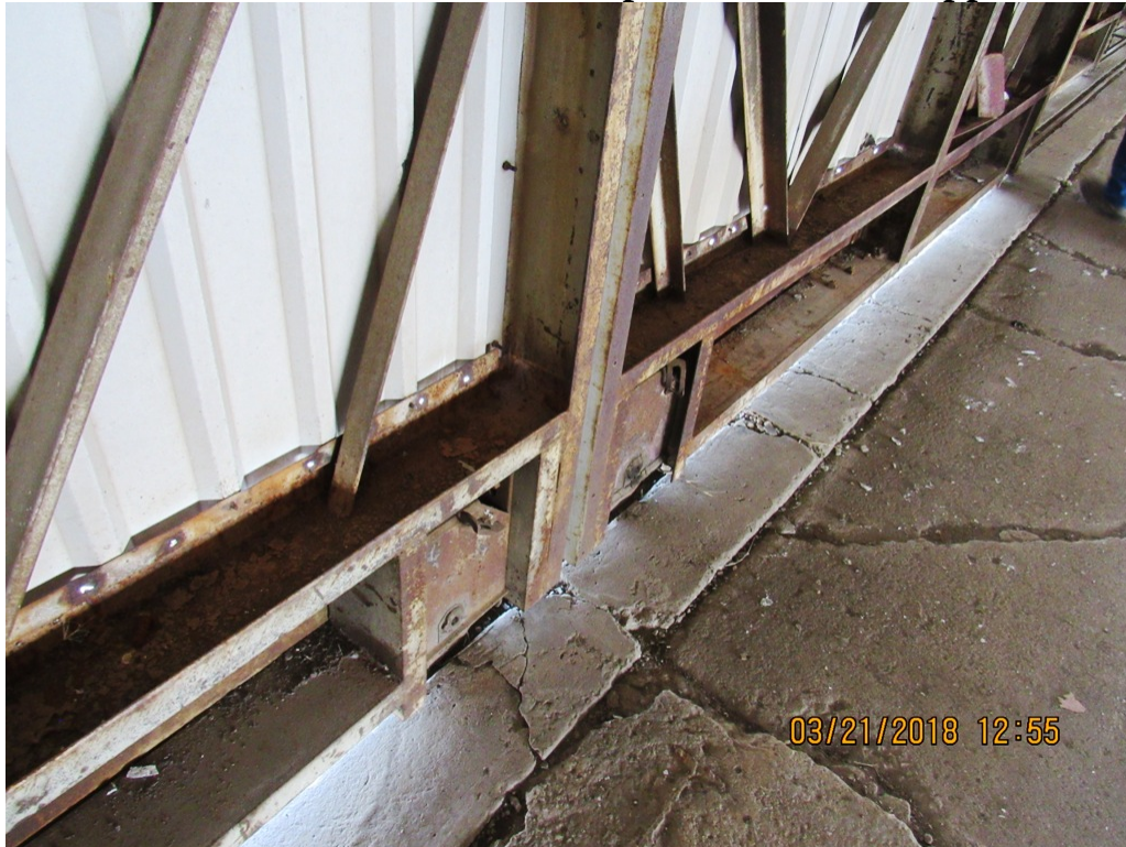
Existing Roller System on Hangar Door
